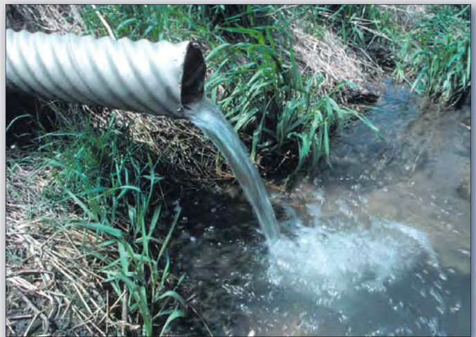
Tile drainage outlet in the watershed.
